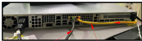
Back view of the Inspextor server
